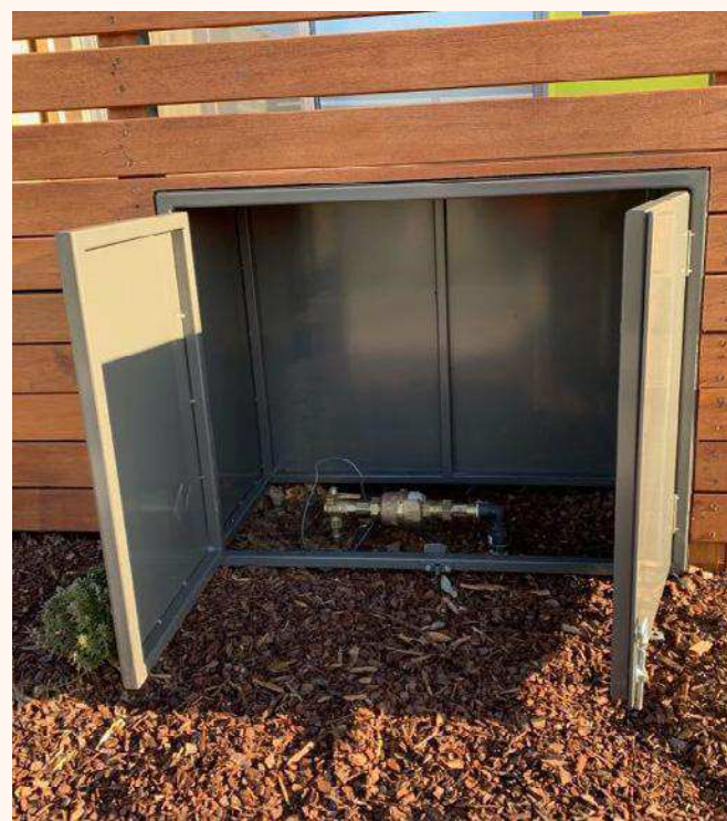
Integrated water meter details within courtyard walls
