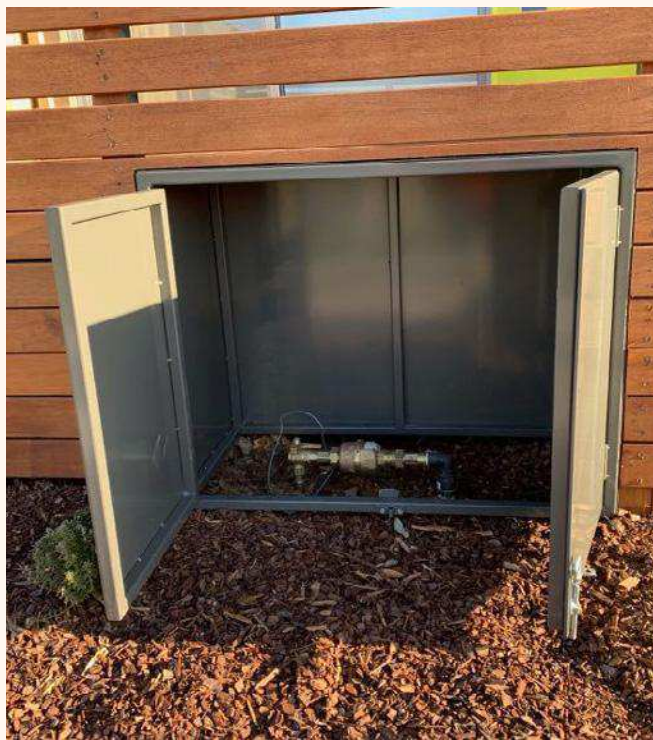
Integrated water meter details within courtyard walls
