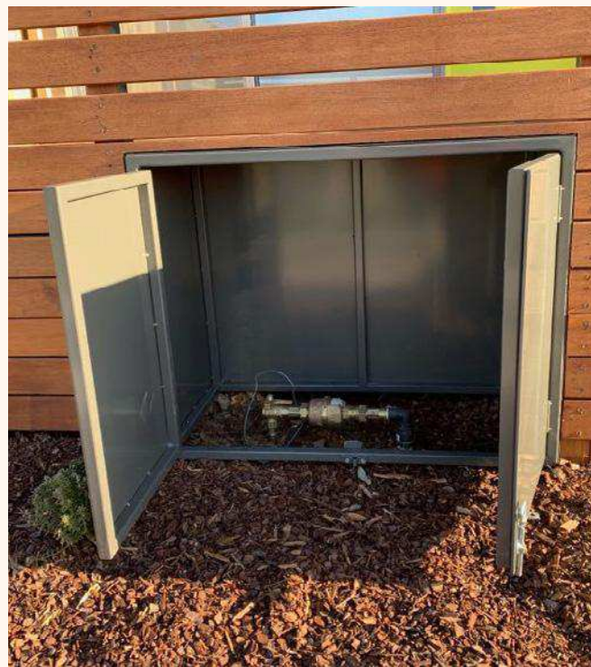
Integrated water meter details within courtyard walls
