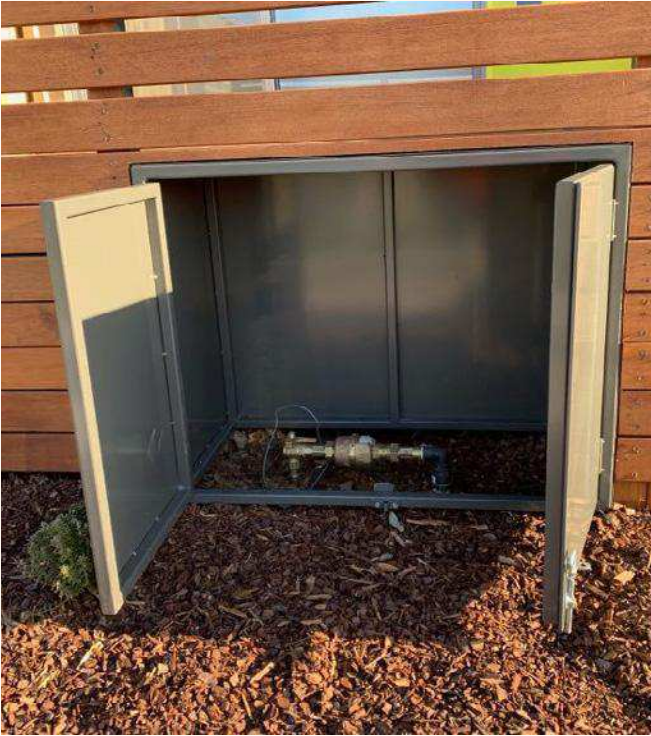
Integrated water meter details within courtyard walls
