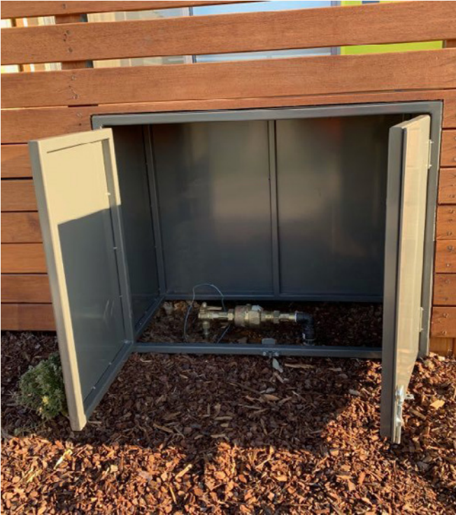
Integrated water meter details within courtyard walls
