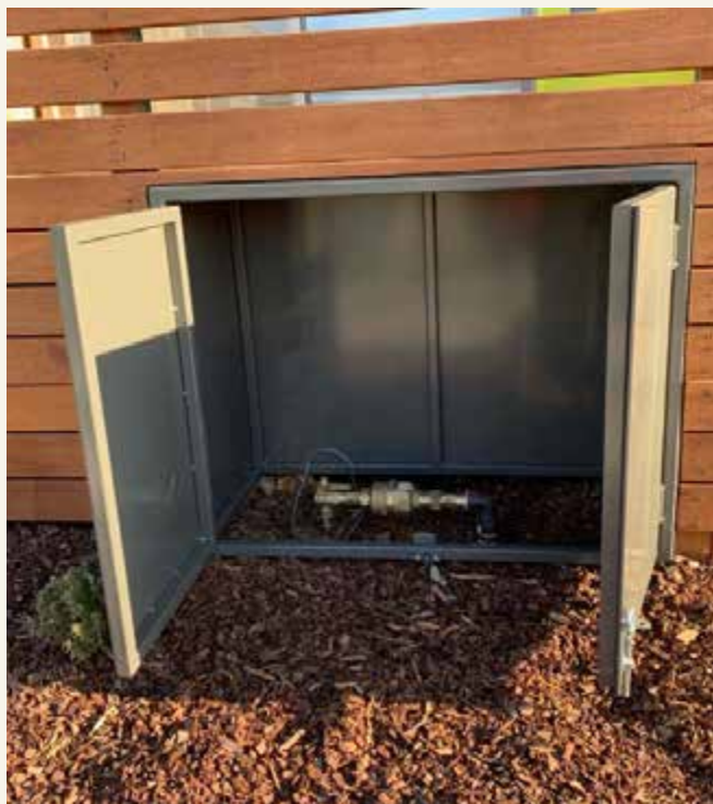
Integrated water meter details within courtyard walls
